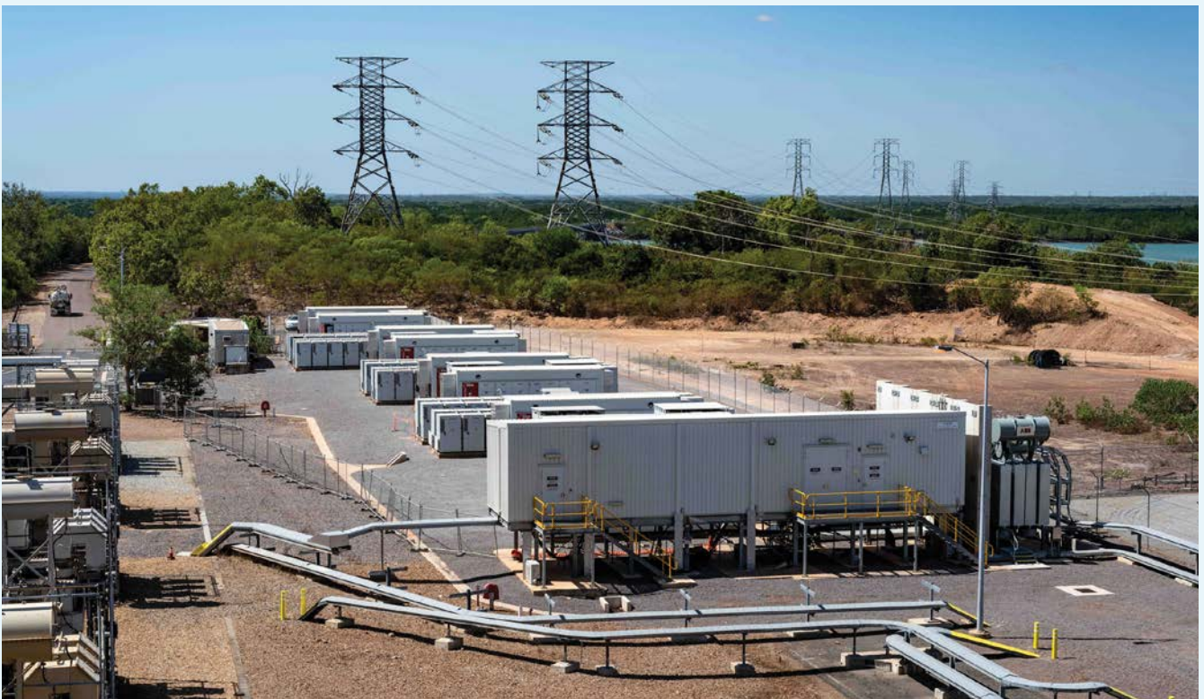
New battery energy storage system on the Darwin-Katherine electricity network. Image credit: Territory Generation.
