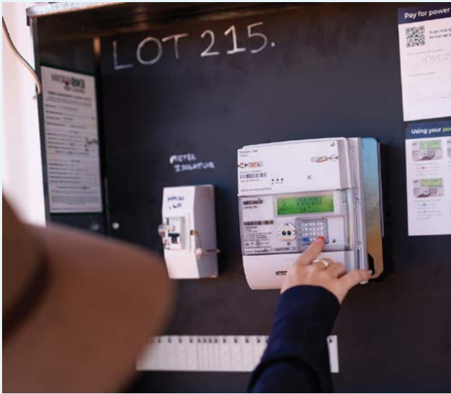
New digital smart meter in Ali Curung.
