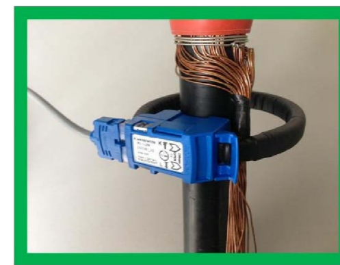
EXAMPLE OF CT INSTALLATION
